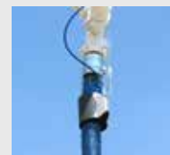
Shut Off valve in pipeline
