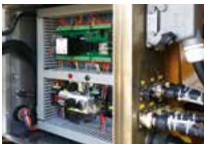
DETACHABLE ELECTRICAL SYSTEM The electrical system can be detached for easy maintenance.
