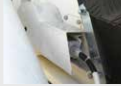
LIMIT SWITCH HOPPER GRID
